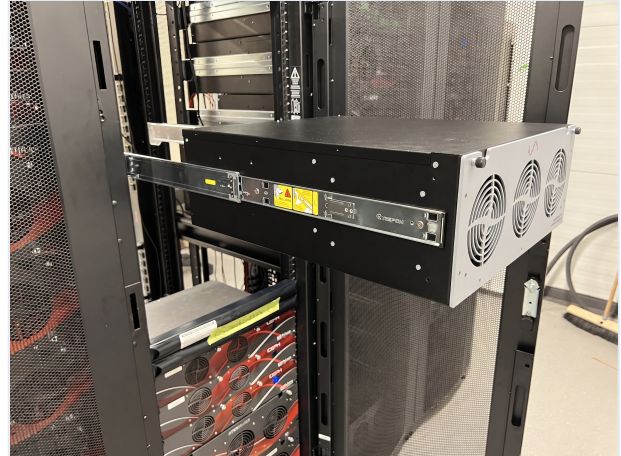
Figure 23: Unit fully racked.
